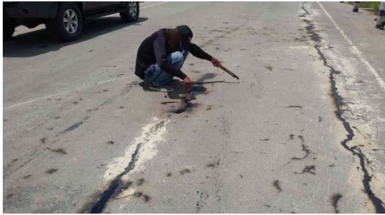
Figure (6): Observation of cracks at the crest of the embankment during excavation
