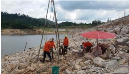
Figure (9): Conduction of bore hole investigation after the movement of the slope in 2014
