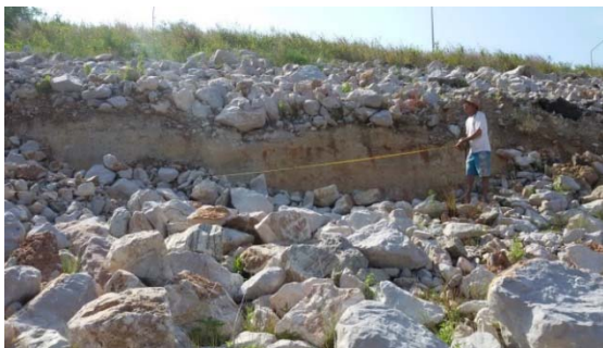
Figure (3): Upstream slope of Pa Bon dam after the first movement
