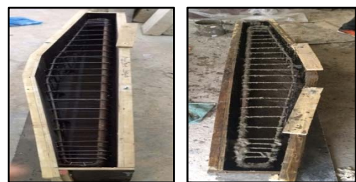
Plate (1): (a) Putting steel reinforcement cage in mold (b) Beam specimen casting
