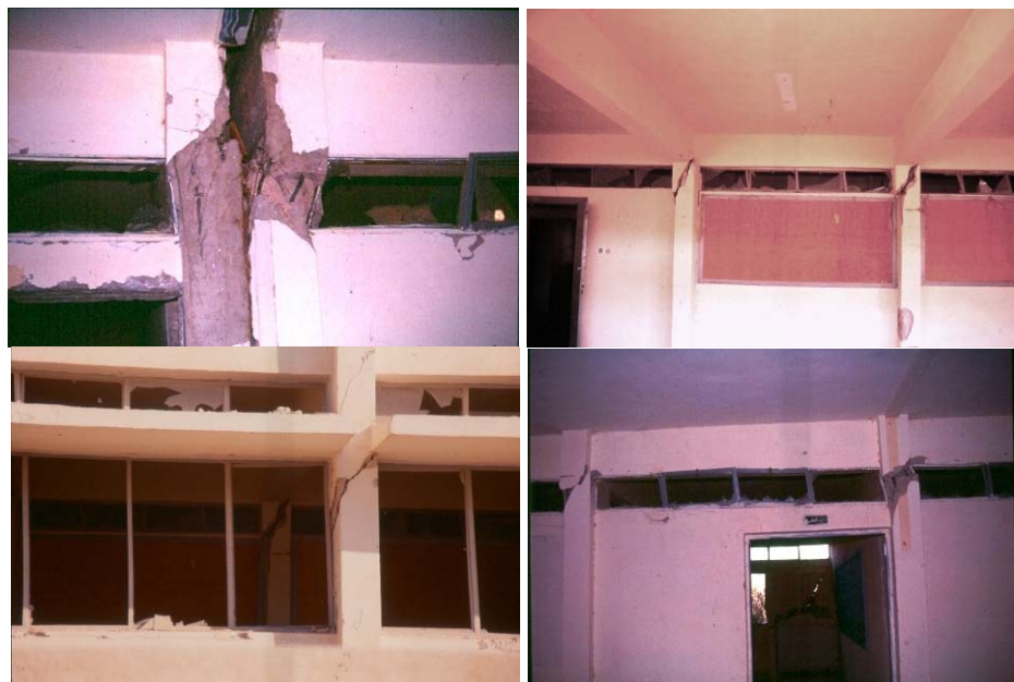
Plate 3: Severely damaged columns of a 2-storey building constructed on expansive soil
