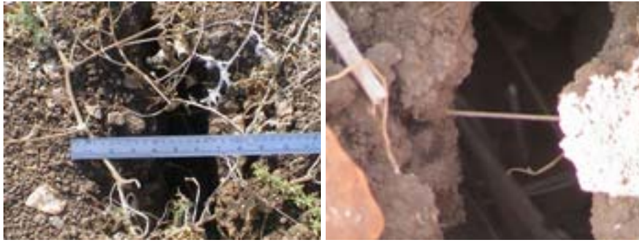
Plate 1: Seventeen cm wide crack in an expansive soil ripping off roots and stretching others
