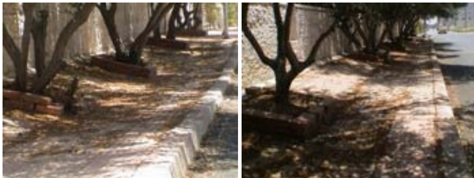
Plate 2: Large deformation caused by bushes in a sidewalk constructed on expansive soil
