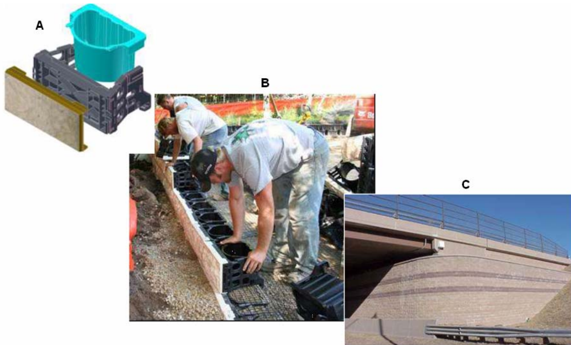
Figure 5: Construction steps of geosynthetic reinforced walls in North America: A) Geosynthetic modular “block” unit components; B) Construction of GRS wall with geosynthetic modular “block” units; and C) Completed bridge abutment
