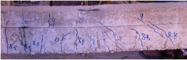
Figure (16)(b): Cracking pattern of specimen GIM-5 (mid-span of the beam)
