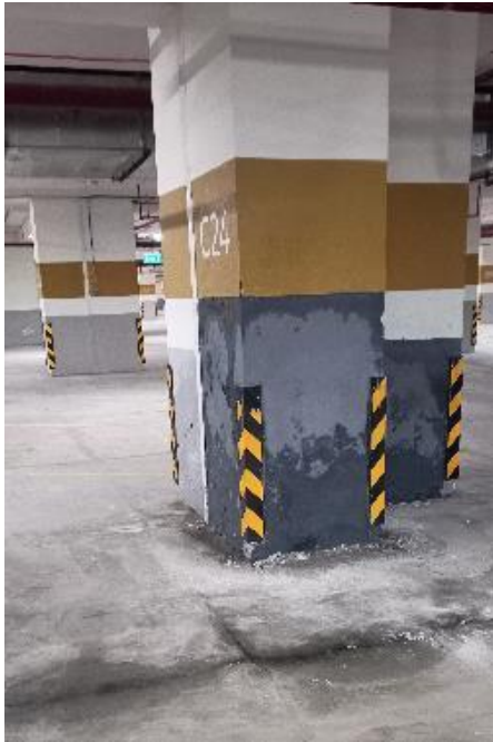
Figure (1): Water leakage in the basement slab of the building
