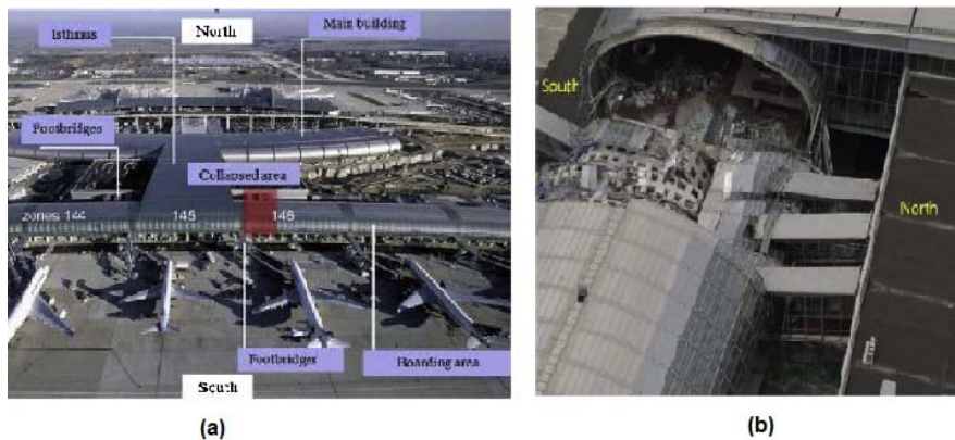
Figure (1): (a) View of the terminal and (b) Collapsed area of the terminal (El Kamari et al., 2015)
