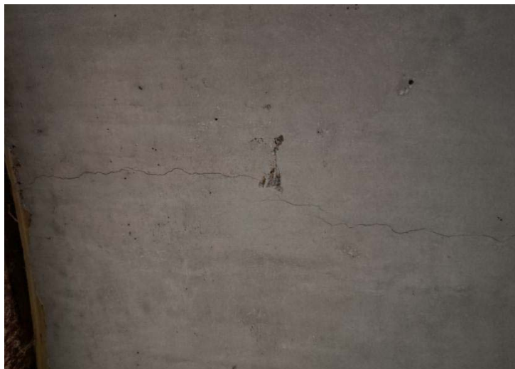
Figure 8. The shape of the crack
