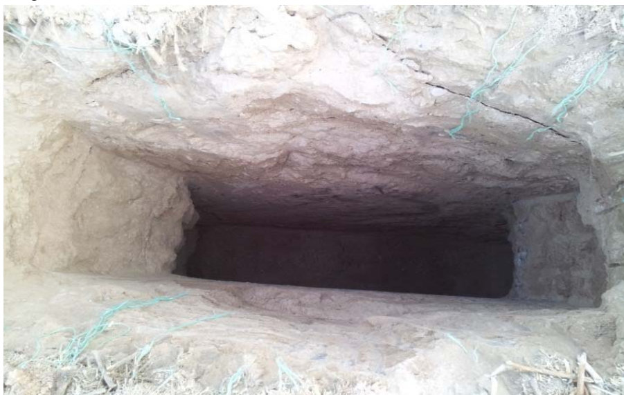
Figure (6): Excavation below ground surface was made to a maximum depth of 2.5 m using a backhole at the studied sites
