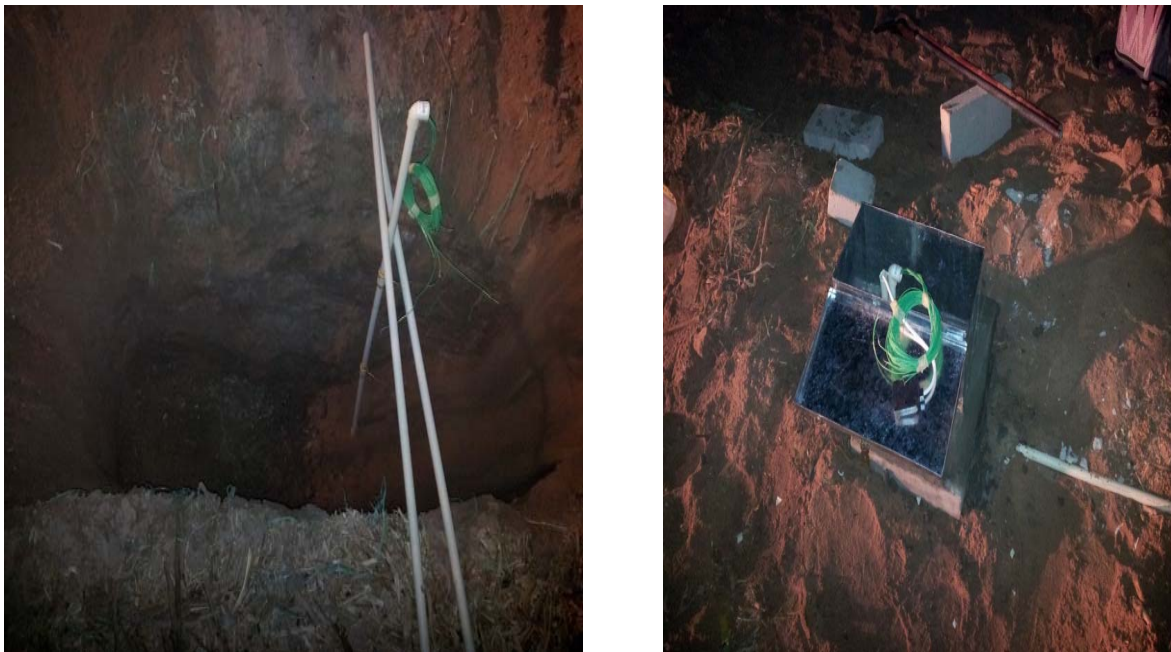
Figure (8): Several flexible sensor wires distributed below ground level to the depth of 2.5 m for measuring and monitoring the sub-soil temperatures
