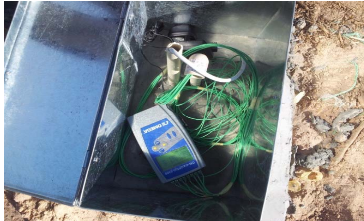
Figure (9): All of the sensors were connected to a data logger that could read and record the measured data for an entire year (≈8760 hours)
