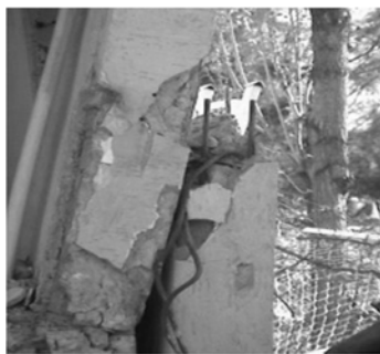
Figure (1): Failure due to insufficient splice length at the top and bottom of the RC column in Bingöl (Turkey) earthquake, 2003 (NISEE)
