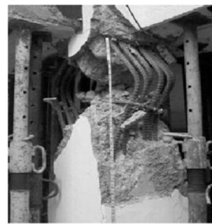
Figure (2): Severe damage in the RC column due to widely spaced transverse reinforcements in Columbia earthquake, 1999 (NISEE)
