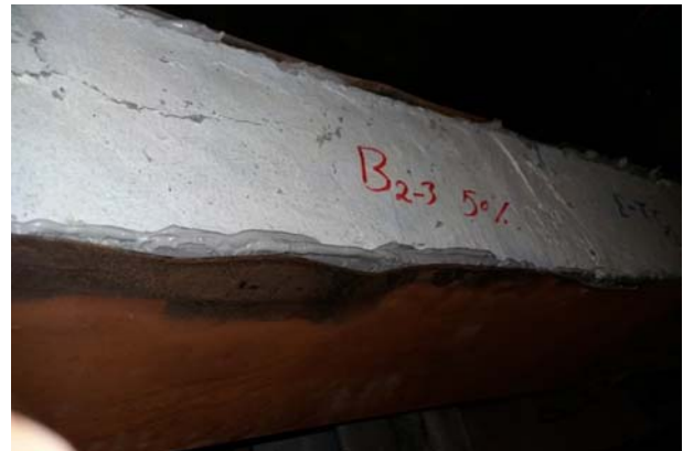
(c) Debonding of steel plates and crushing of concrete at the load points of beam B2-3
