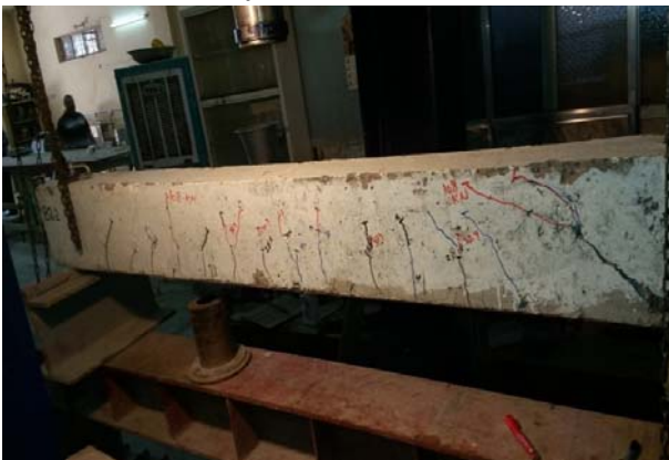
(b) Flexural and shear failure of beam B2-2
