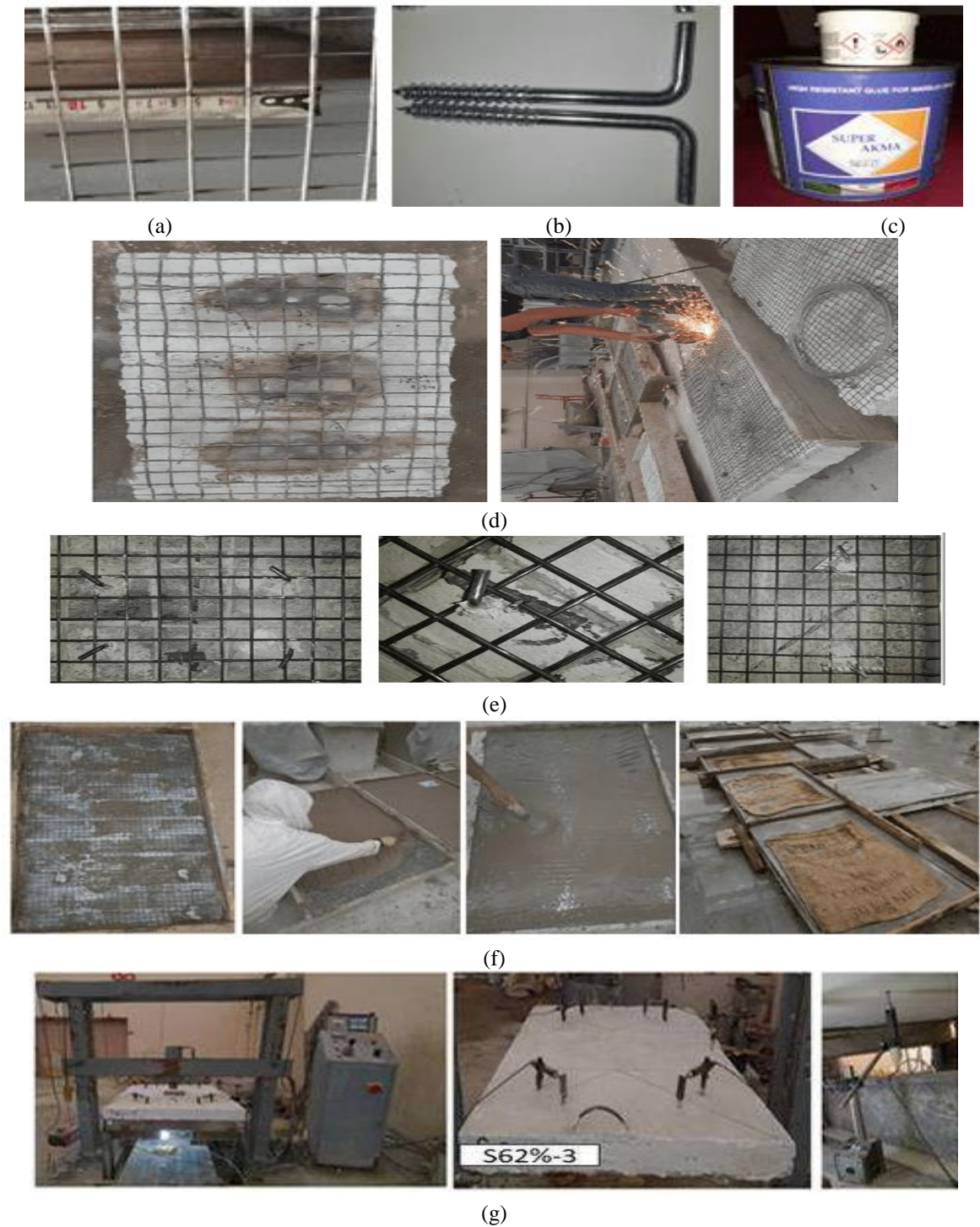
Figure (3): (a) Metal mesh, (b) Bolts, (c) Polyester maleate, (d) Roughing surface, (e) Location of bolts, (f) Repairing process and (g) Loading device and sensor locations
