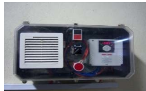
Figure (2): Frequency-adjusting device used to control flow rate
