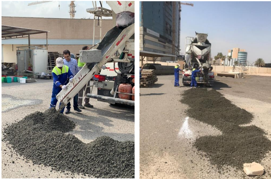
Figure (1): Extraction of granular aggregates (a) discharge of treated aggregates and (b) spreading for adequate curing
