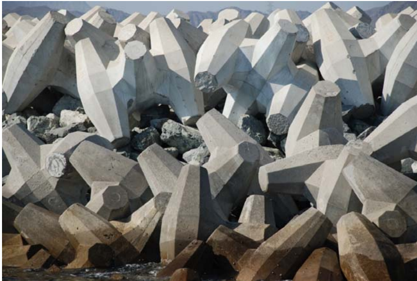
Figure (4): Movements of concrete armour units with large settlements [Source: Hendrikse, 2014]
